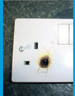
Typical examples of potentially dangerous electrical installations
